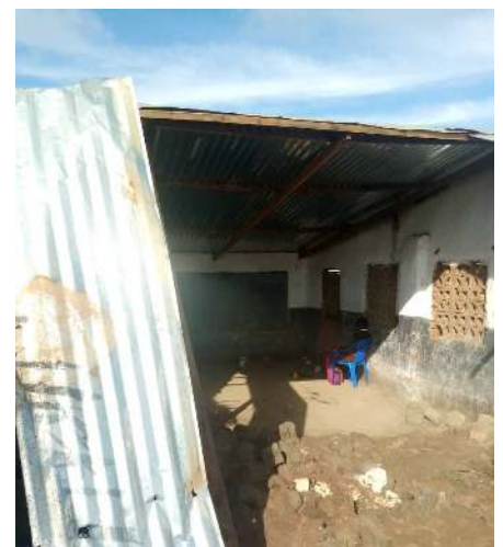
The classroom has since partially collapsed
