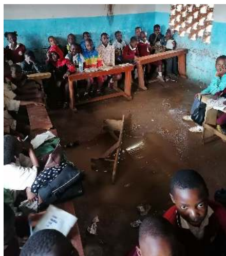
A pool of water in the classroom - the roof was letting in
